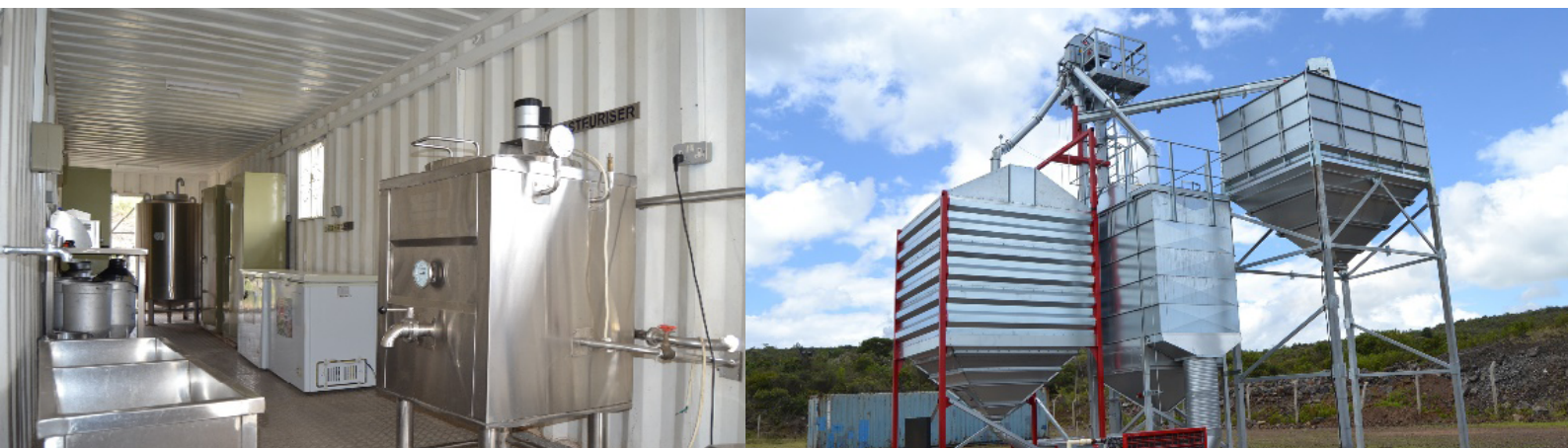
Photograph 5: Menengai direct use project: Milk pasteuriser (left) and grain dryer (right)
